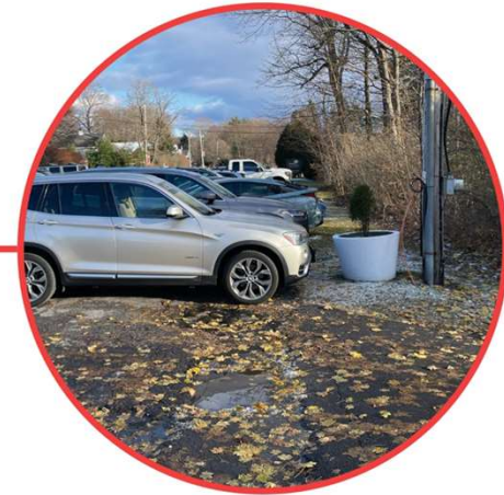
Cars parked with varying depths, resulting in inconsistent drive aisle width and vehicle overhang
